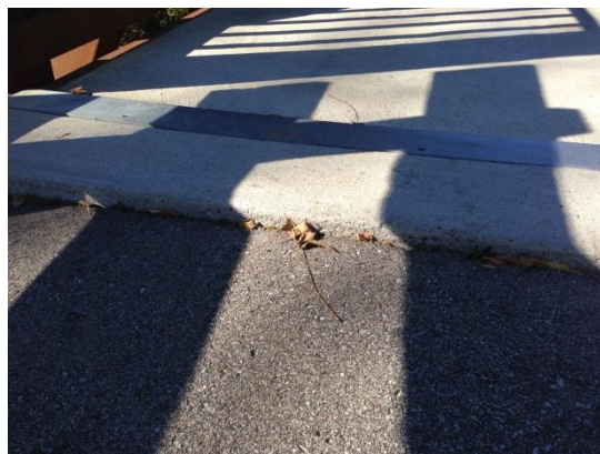
Photos this page (clockwise from top left): Interpretive signage along trail; Area of trail with erosion; Monon Trailhead location where crack exists from settling; Transition Lip on Bridge; Bent sign along Monon Trailhead location
